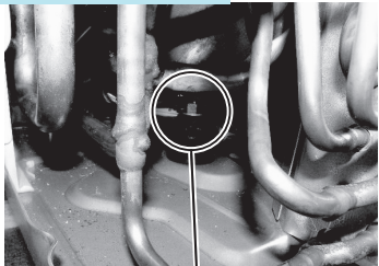
Nut of compressor fixing bolts
